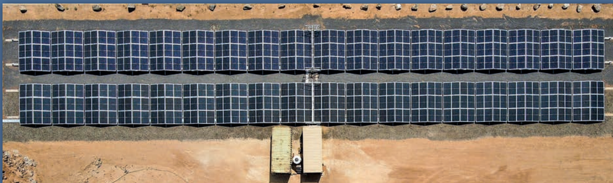
Kapi hybrid and deployable power plant for isolated sites, copyright Kapi
